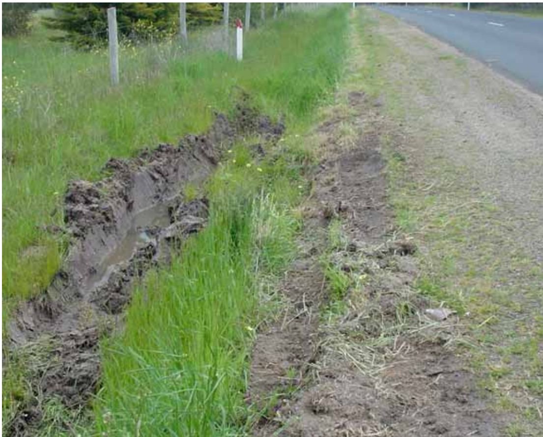
Figure 9. Rutting caused by roadside slashing
